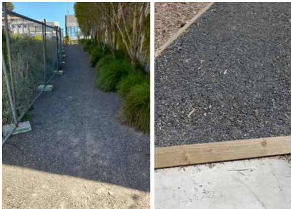
Unsafe upper path
