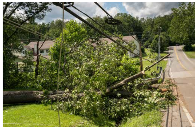
Power and telecommunications infrastructure often runs parallel with roads, so is vulnerable to slips and landslides.
