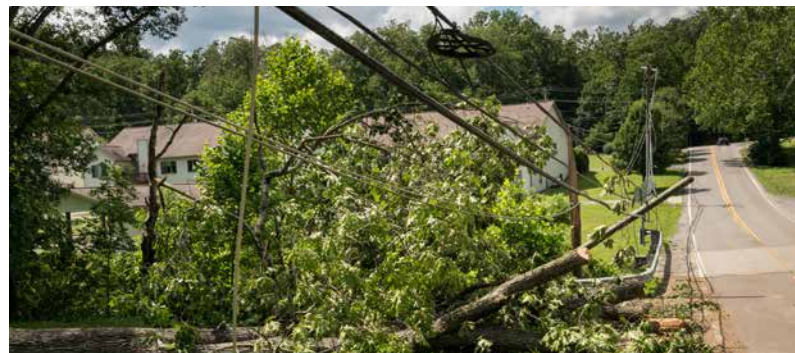
Power and telecommunications infrastructure often runs parallel with roads, so is vulnerable to slips and landslides.
